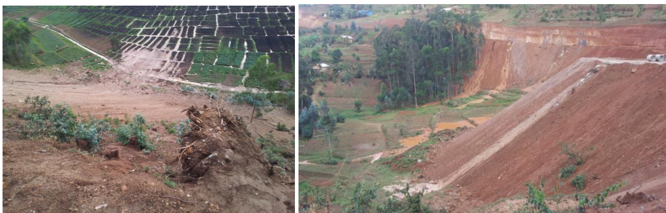
FIGURE 2-72: Gravel road non-point source pollution above valley-bottom wetlands during construction of Base-Butaro-Kidaho road
