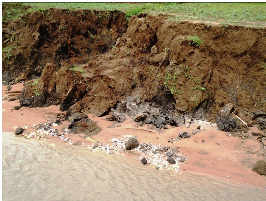
FIGURE 4-3 Example of river bank collapse from erosion next Nyarububa wetland, Rulindo District
