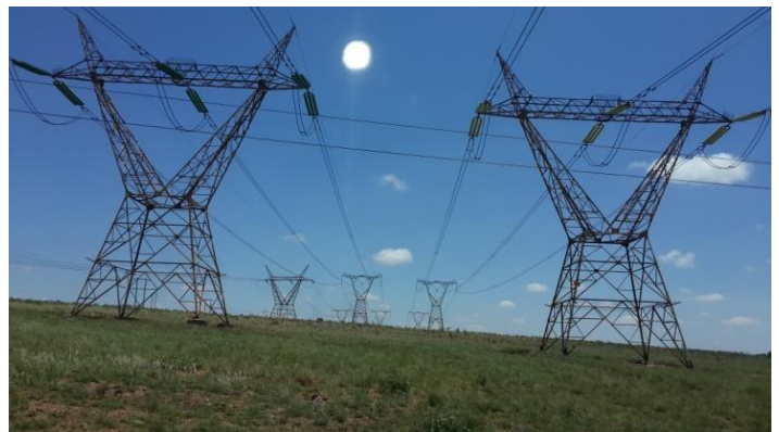
Eskom power lines traverse the site. On northern boundary.
