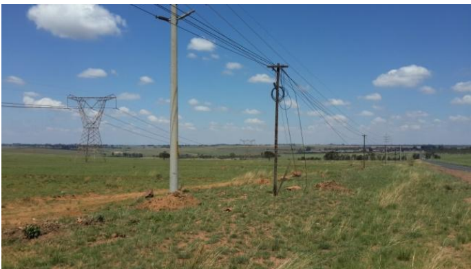
Eskom power lines traverse the site. Along the R544
