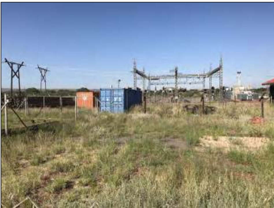
Figure 23: Typical view of the Segame Substation
