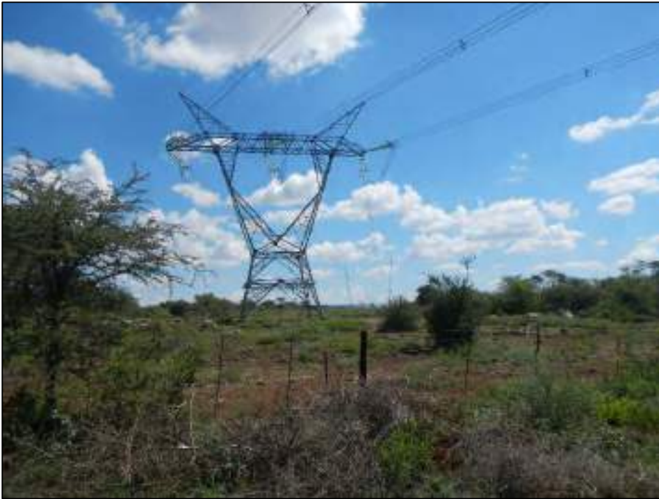
Figure 22: Typical view of the Ferrum-Mercury 400kV transmission power lines which traverse the study area
