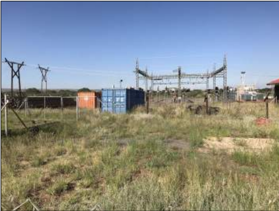
Figure 25: Typical view of the Segame Substation
