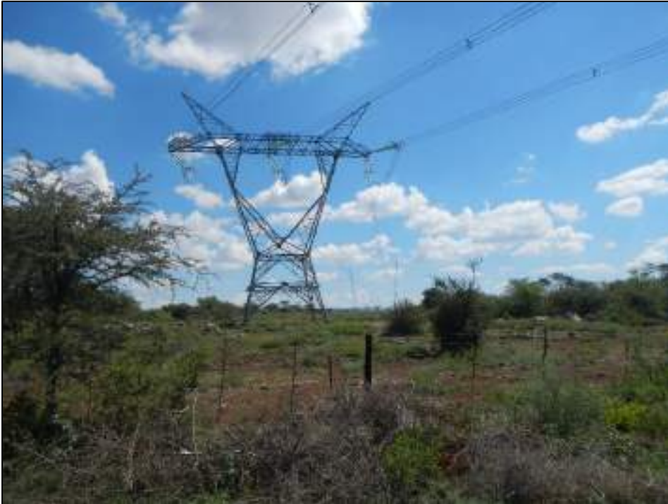
Figure 23: Typical view of the Ferrum-Mercury 400kV transmission power lines which traverse the study area
