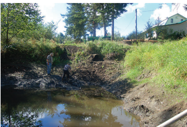
The culvert looking downstream. Note the height of the culvert above the water.
