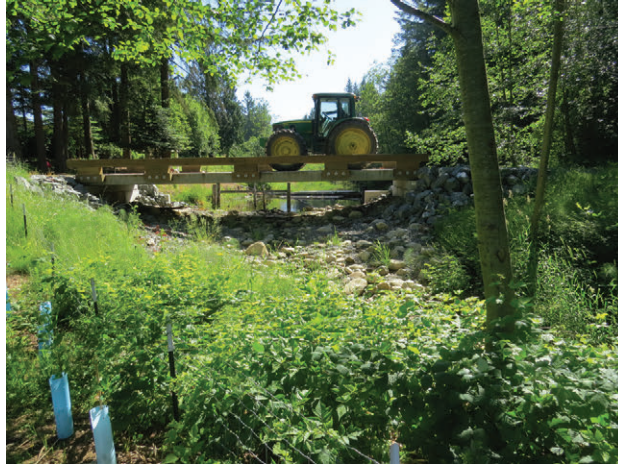
The bridge is more reliable than the old road that went over the culvert, and can accommodate our heavy machinery. Photo credit: Todd Jones
